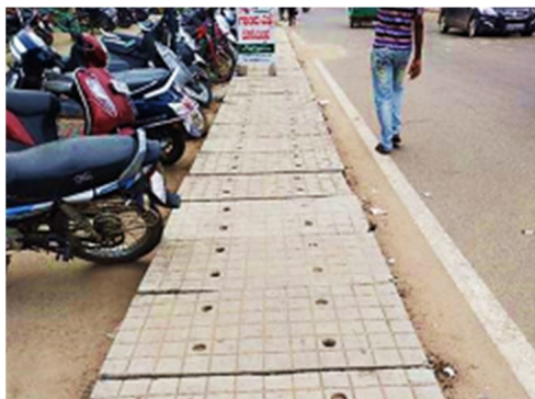
Figure 10:Drain covering as <1m footpath Source: Author
