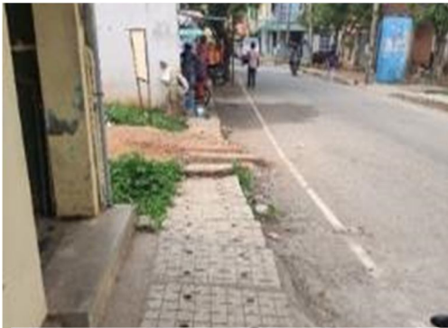
Figure 25: Discontinuous footpath Source: Author
