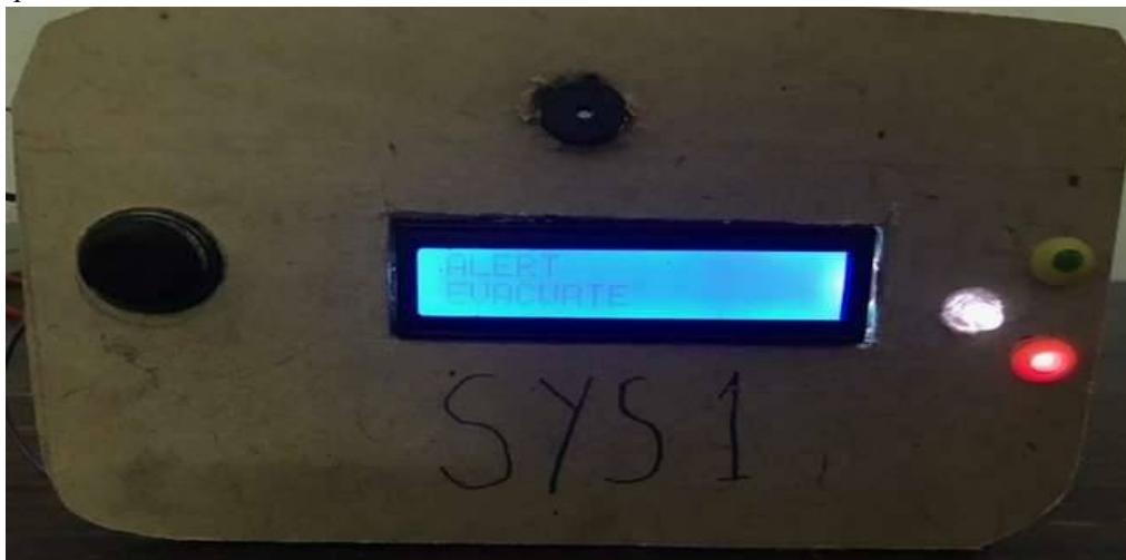
Figure 10.2 Gas detector 1 during gas leak scenario
