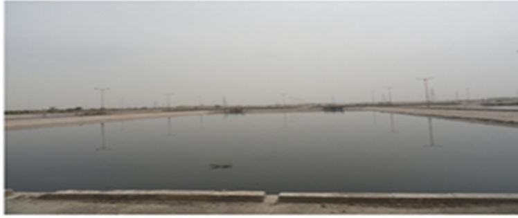
SECOND ANAEROBIC STABILIZATION POND, BIKANER
