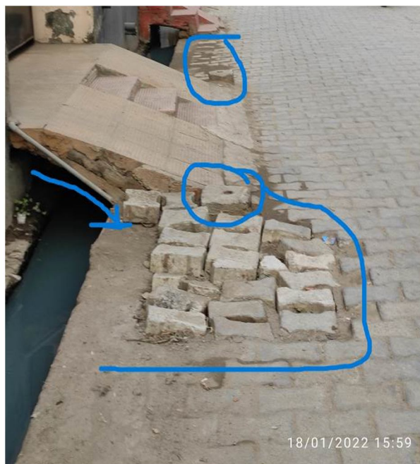
Figure 19 Encroachment and illegal construction
