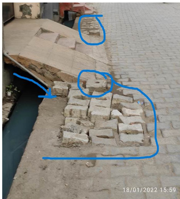
Figure 19 Encroachment and illegal construction
