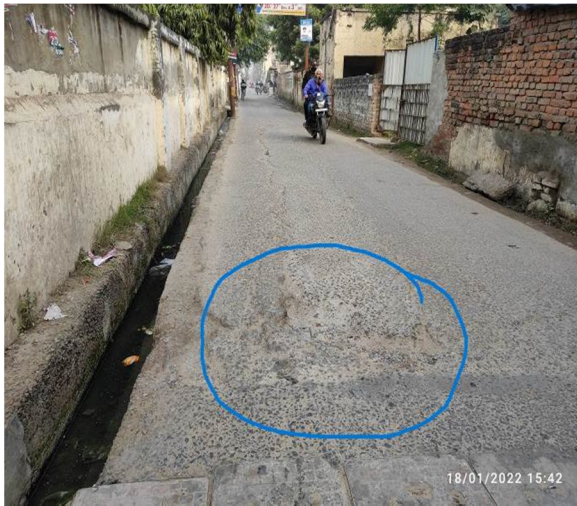
Figure 13 Eroded encasement surfaces
