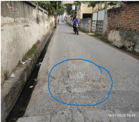
Figure 13 Eroded encasement surfaces
