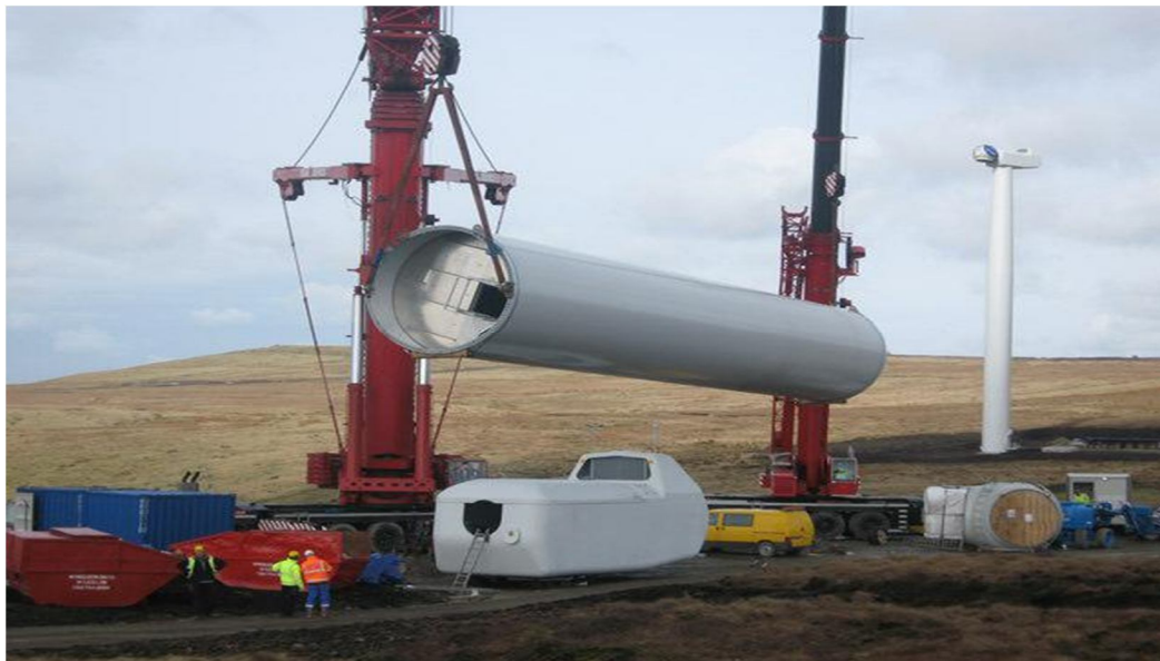
Figure.1. OSH risks associated with the construction of wind turbines (Unloading of Tower cells)
