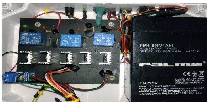
Fig. 4 Power Supply Unit of the System
