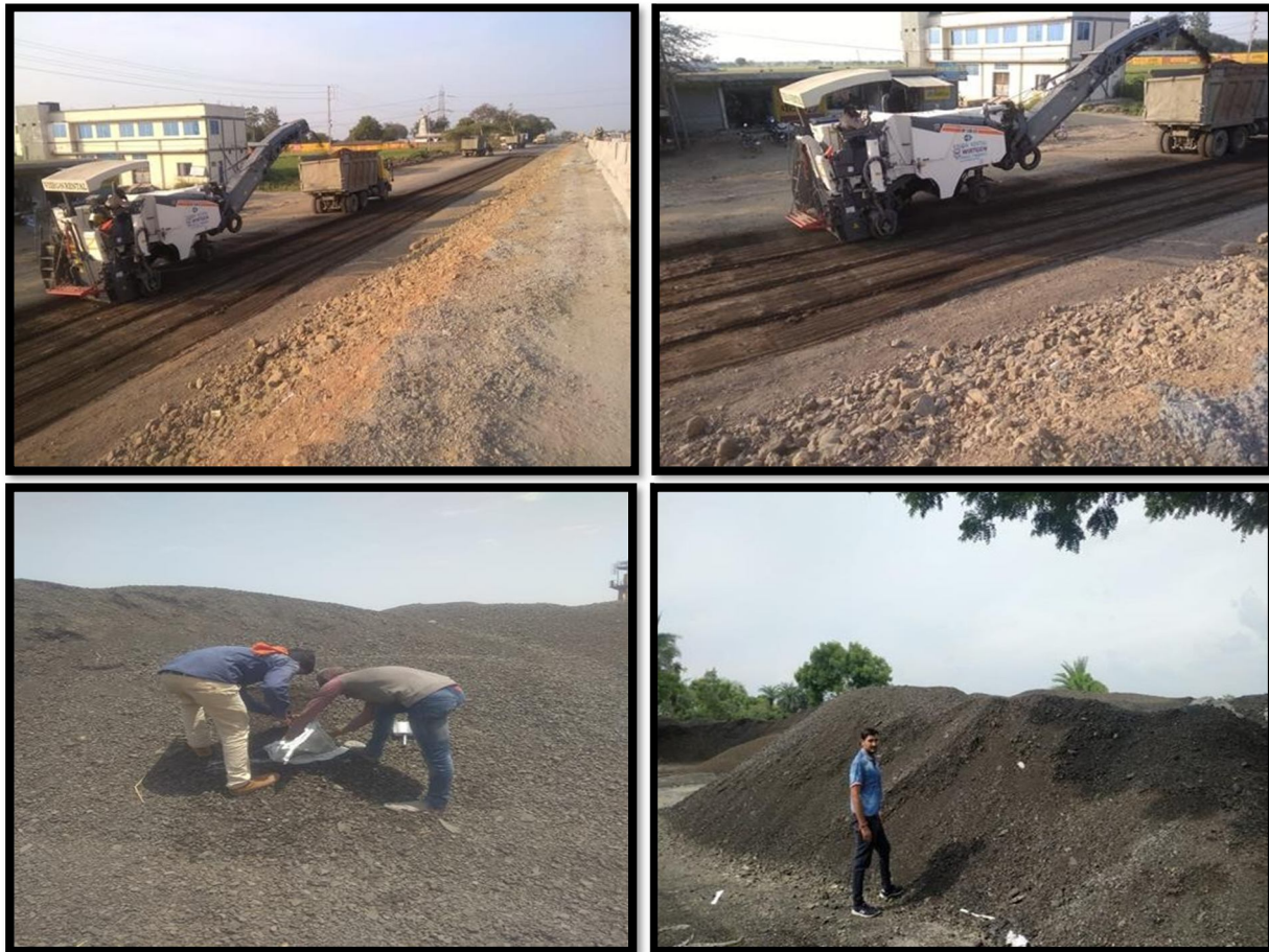
Figure-: Milling of existing bituminous layer at site & Sampling of material from stockpile
