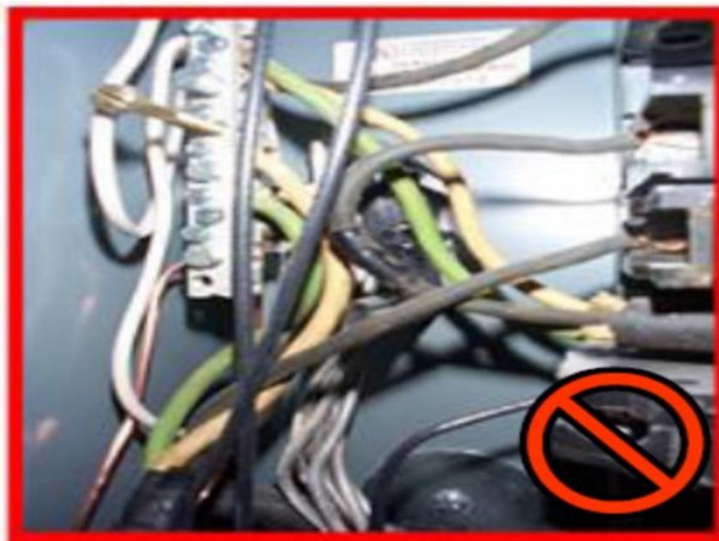
Fig no: 4.1 Exposed Electrical Parts
