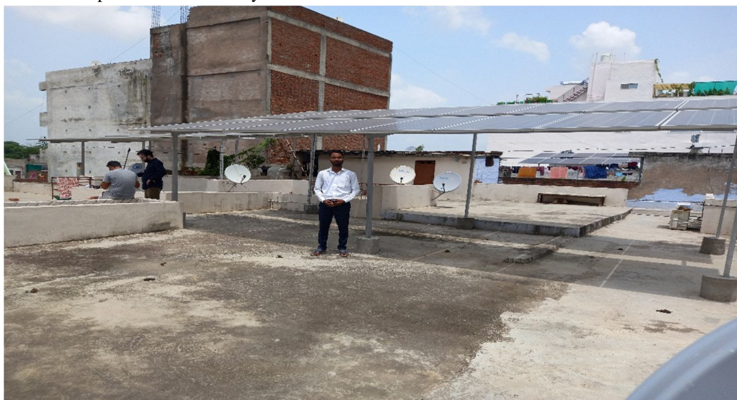
Figure 5. Solar Rooftop Photovoltaic System (RTPV I)
