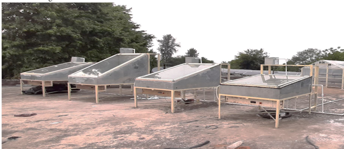
Fig.2 Solar stills installed on MITS Roof
