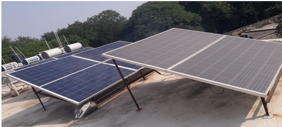
Fig.1 PV Solar setup on roof of MITS Gwalior
