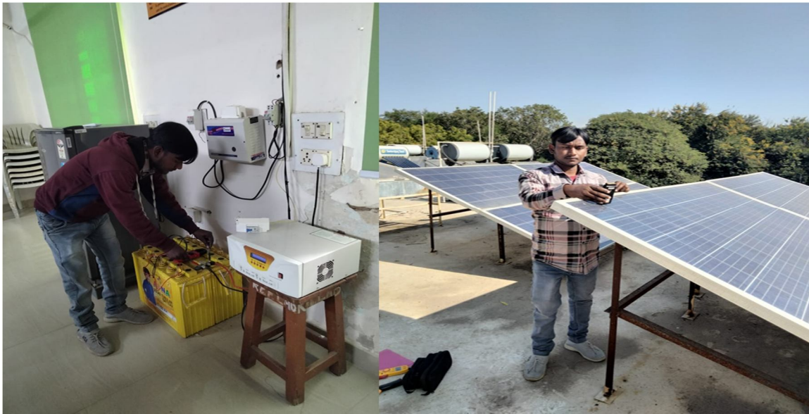
Fig 5 Photograph of PV panel and Battery – Inverter Arrangements
