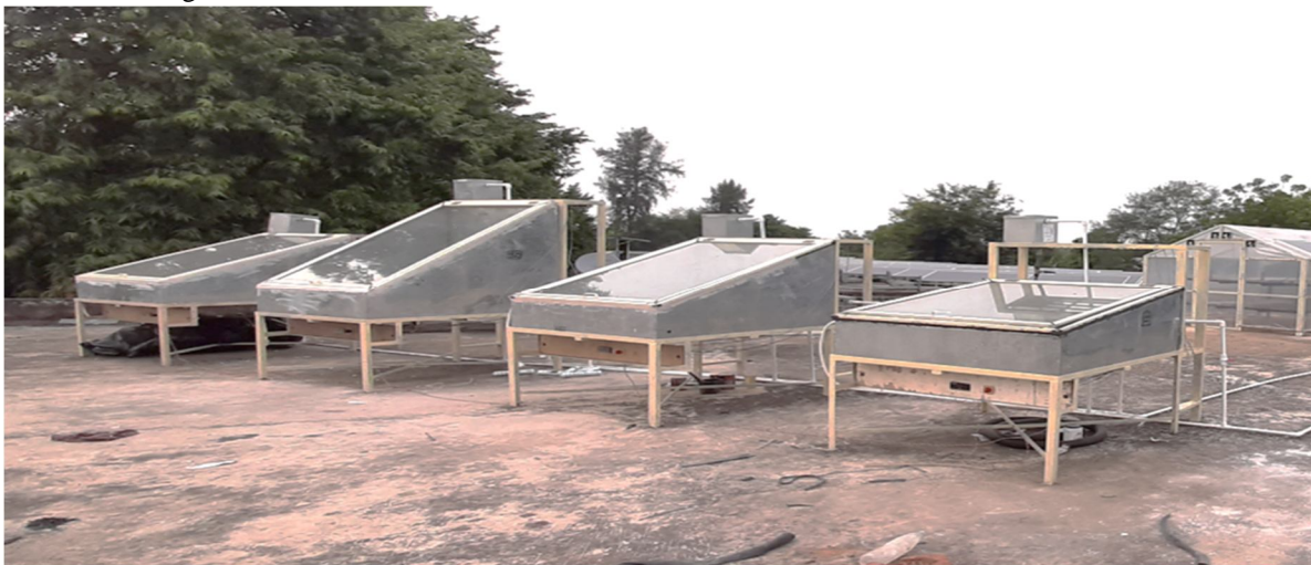
Fig.2 Solar stills installed on MITS Roof
