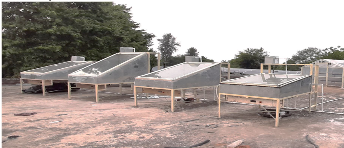
Fig.2 Solar stills installed on MITS Roof
