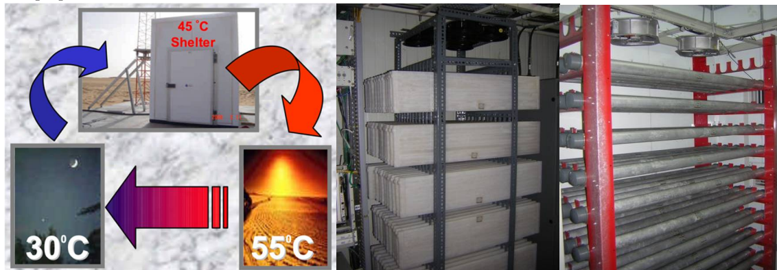
Fig 11. Thermal management in telecom shelters using HDPE panels and aluminum pipes filled with PCM and stacked neatly.
