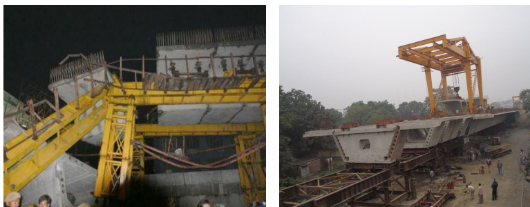
Fig 5.1: (a) Hyderabad Flyover accident in 2007 due to failure of staging. (b) Ground supported launching arrangement before staging failure on NH-16.
