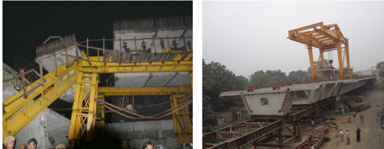
Fig 5.1: (a) Hyderabad Flyover accident in 2007 due to failure of staging. (b) Ground supported launching arrangement before staging failure on NH-16.
