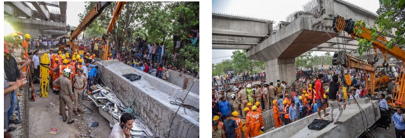
Fig 1.2:- Varanasi UP Flyover Girders collapse on 15-May-2018
