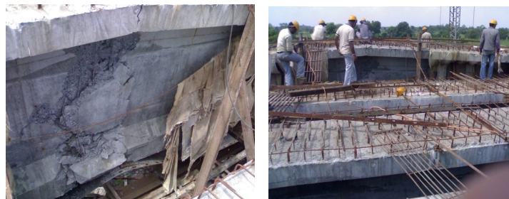
Fig 3.1:- Crushing of concrete at weak flexural zone due to insufficient conc strength
