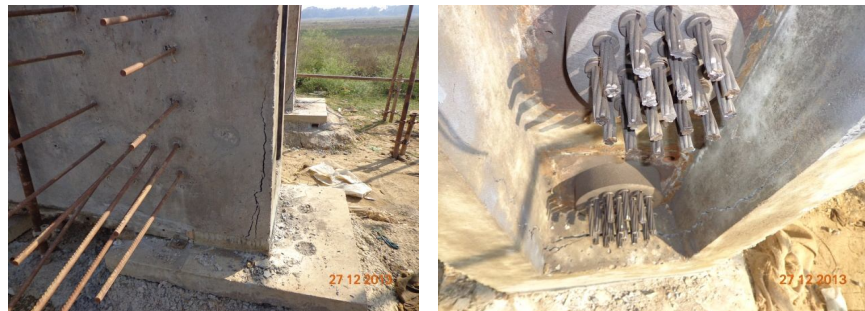
Fig 4.1:- Removal of Girder Concrete skin due to Rigid casting bed at End Block portion.
