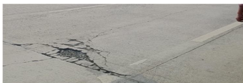
Spalling at cracks
