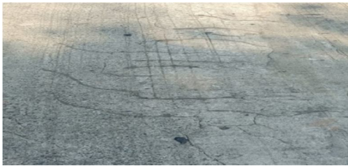
Plastic Shrinkage Cracks
