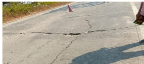
Multiple Structural Cracks
