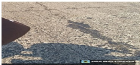
Loss of surface Texture, polished surface
