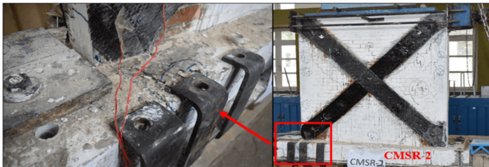
Figure 10. Crack pattern and failure mode after Retrofitting
