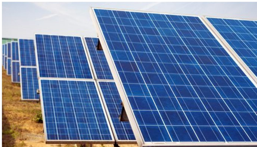
Fig.9. – Array of Solar Cells and Panels for Smart Energy System
