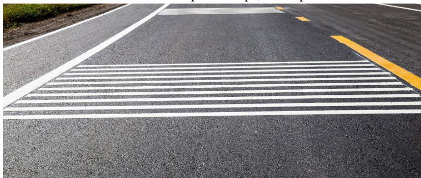
Fig.8 Rumble along the length of road at midway.
