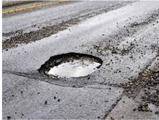
Figure 1: A pothole in the middle of the road.
