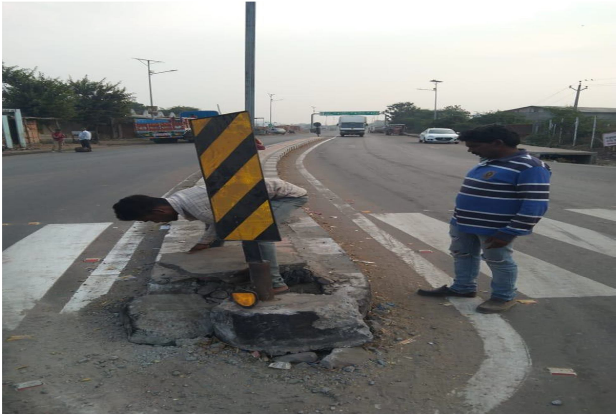
Ch. 0+010 Damaged delineator sign board should be changed & median side kerb should be repaired.
