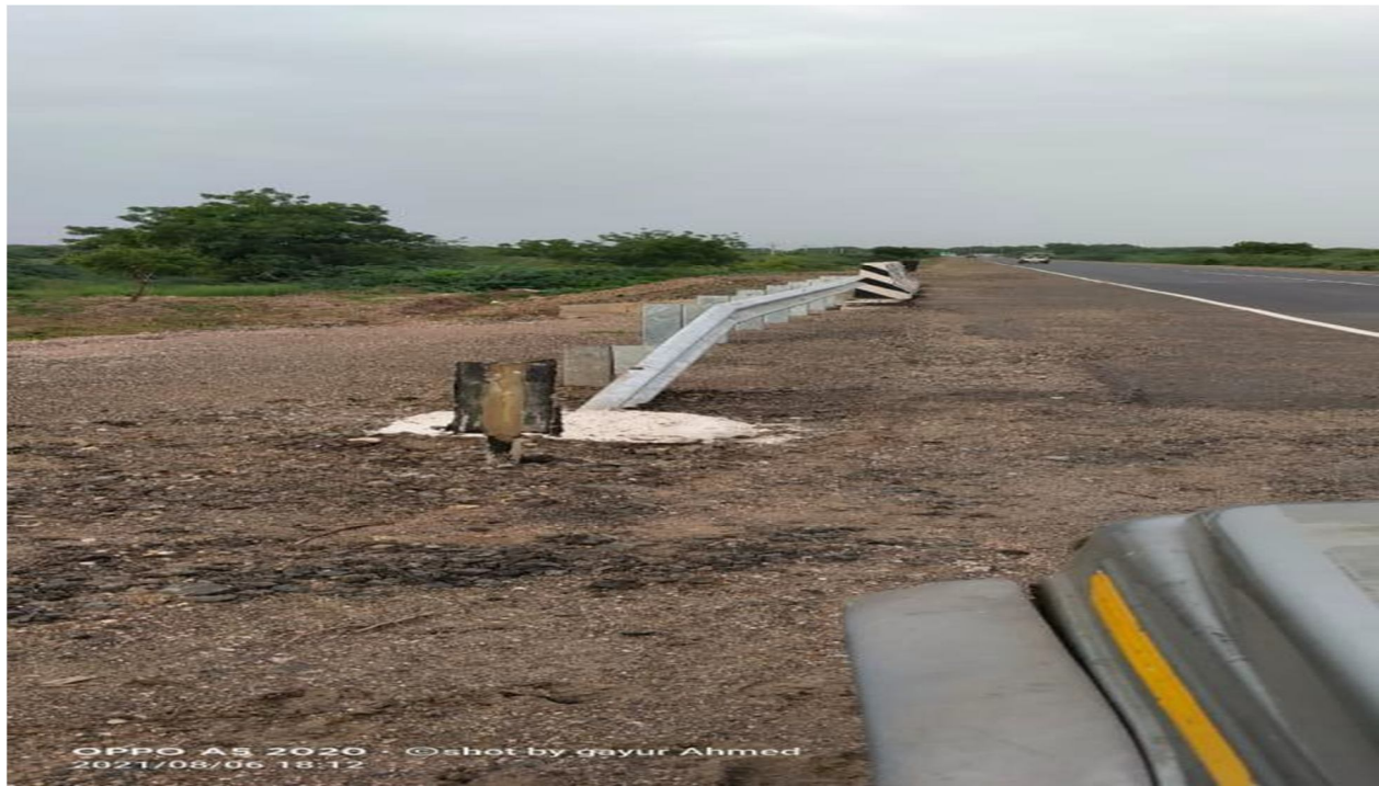
Ch. 7+700 Hazard marking sign board found damaged & faded condition
