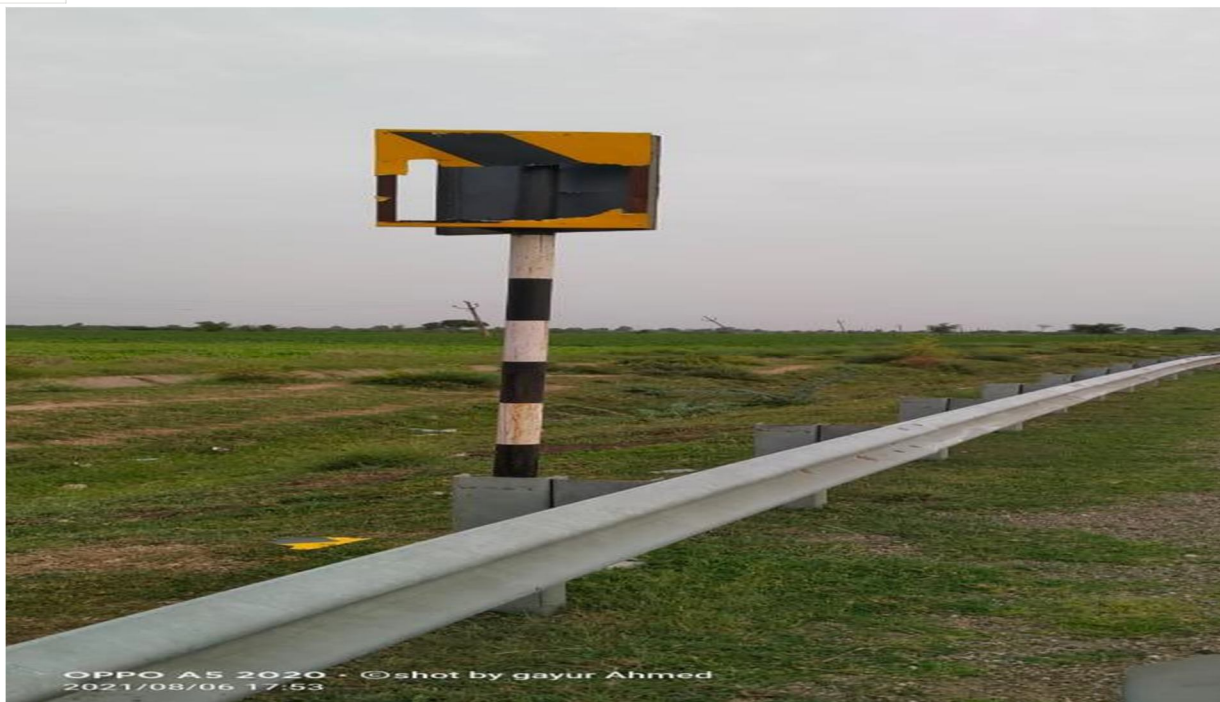
Ch. 16+440 Right hand chevron sign board found in damaged condition
