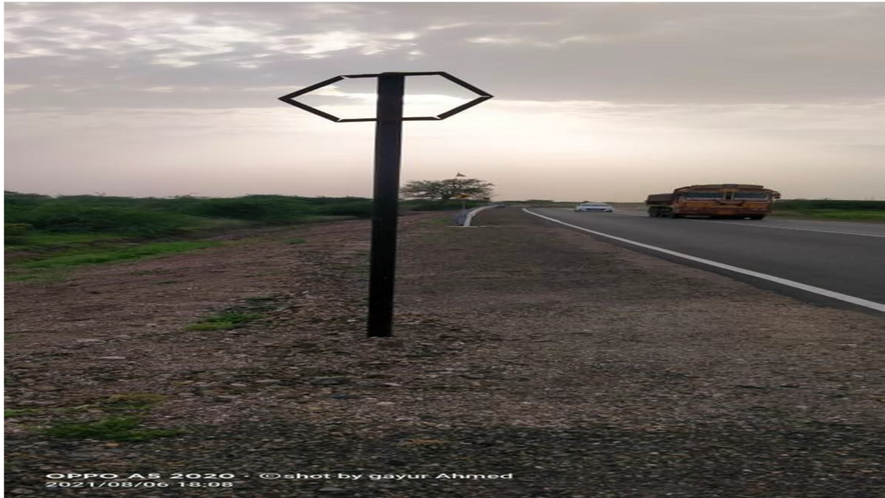
Sign board found damaged at Ch. 7+290
