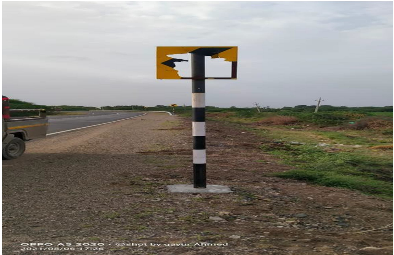
22+300 Left turn chevron sign board found in damaged condition
