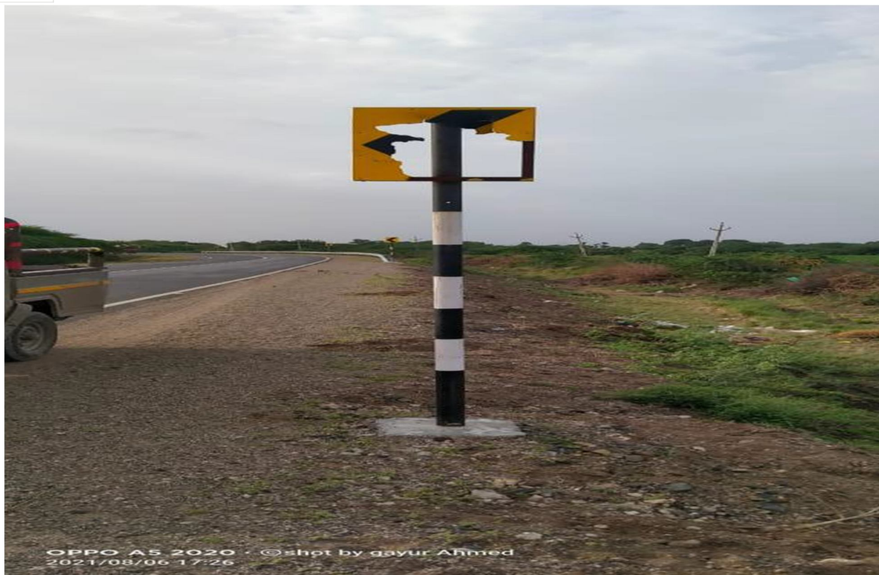
22+300 Left turn chevron sign board found in damaged condition
