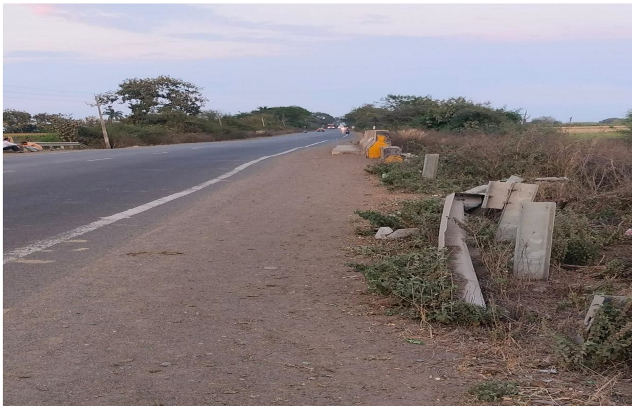
Ch. 15+750 Metal Beam Crush Barrier (MBCB) damaged must be repaired
