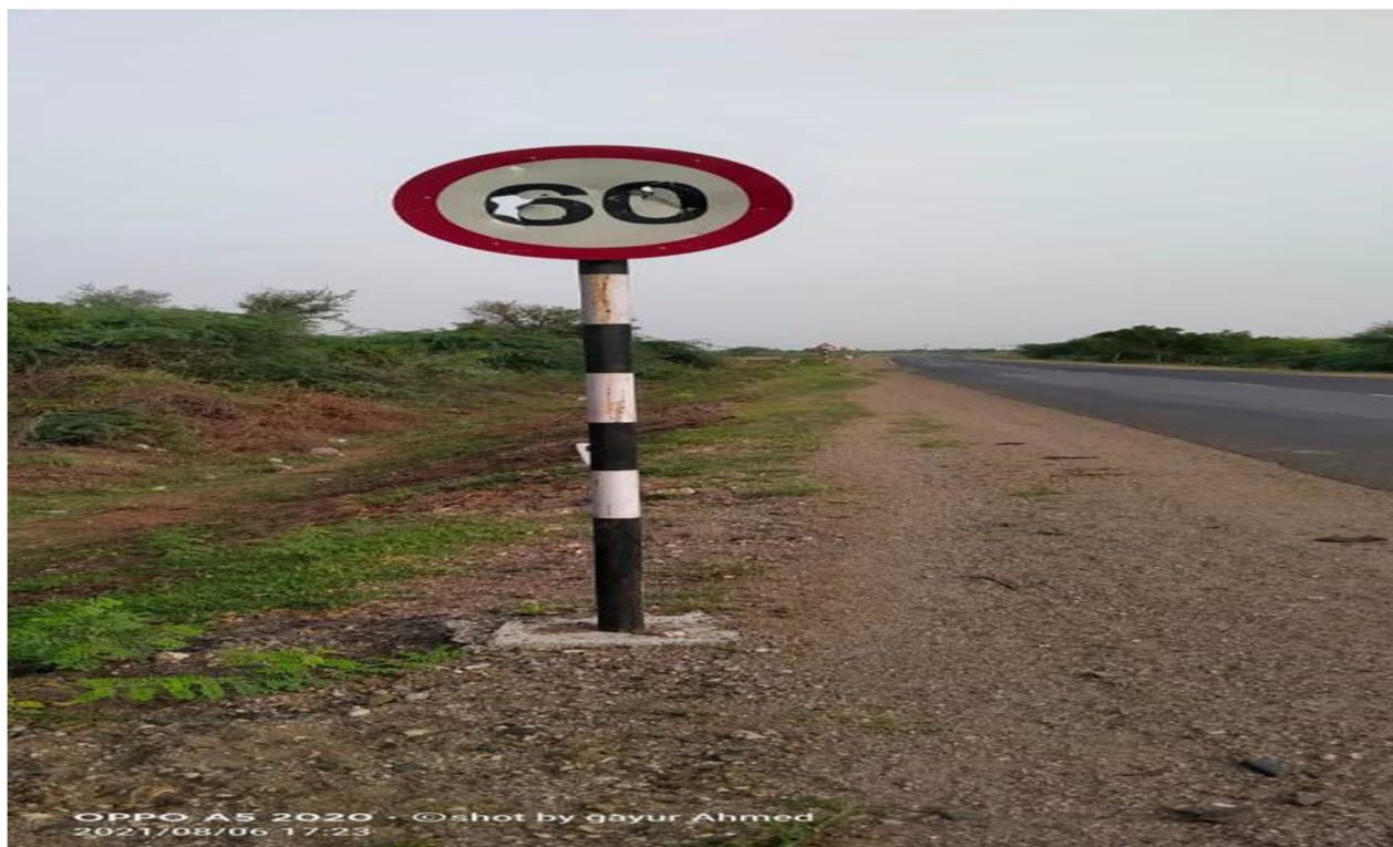
Ch. 26+500 Damaged speed limit sign board
