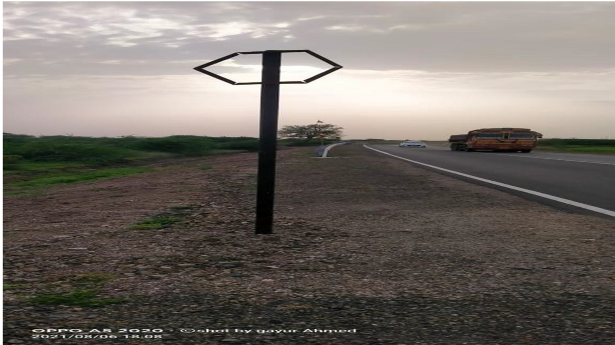
Sign board found damaged at Ch. 7+290
