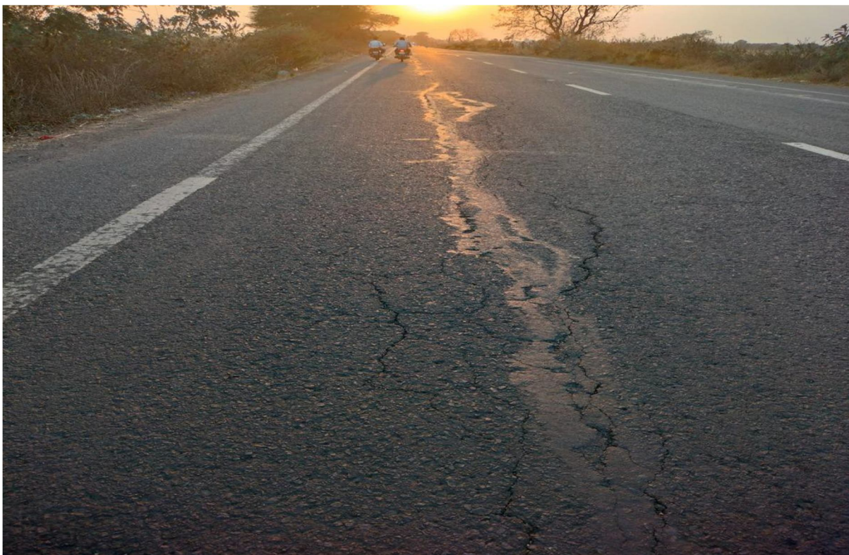
Ch. 3+530 Alligator cracking is observed on Pavement Surface
