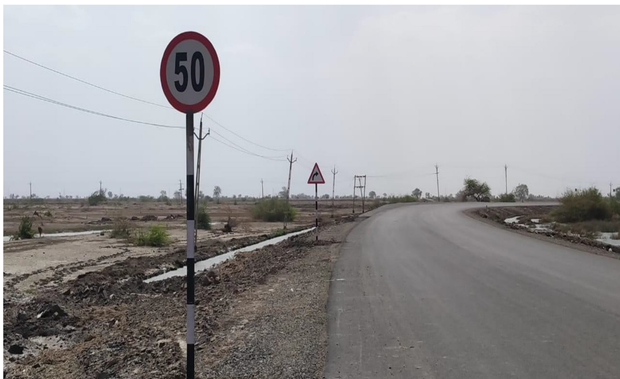
Ch. 20+900 Missing road marking & rain cuts observed near earthen shoulder
