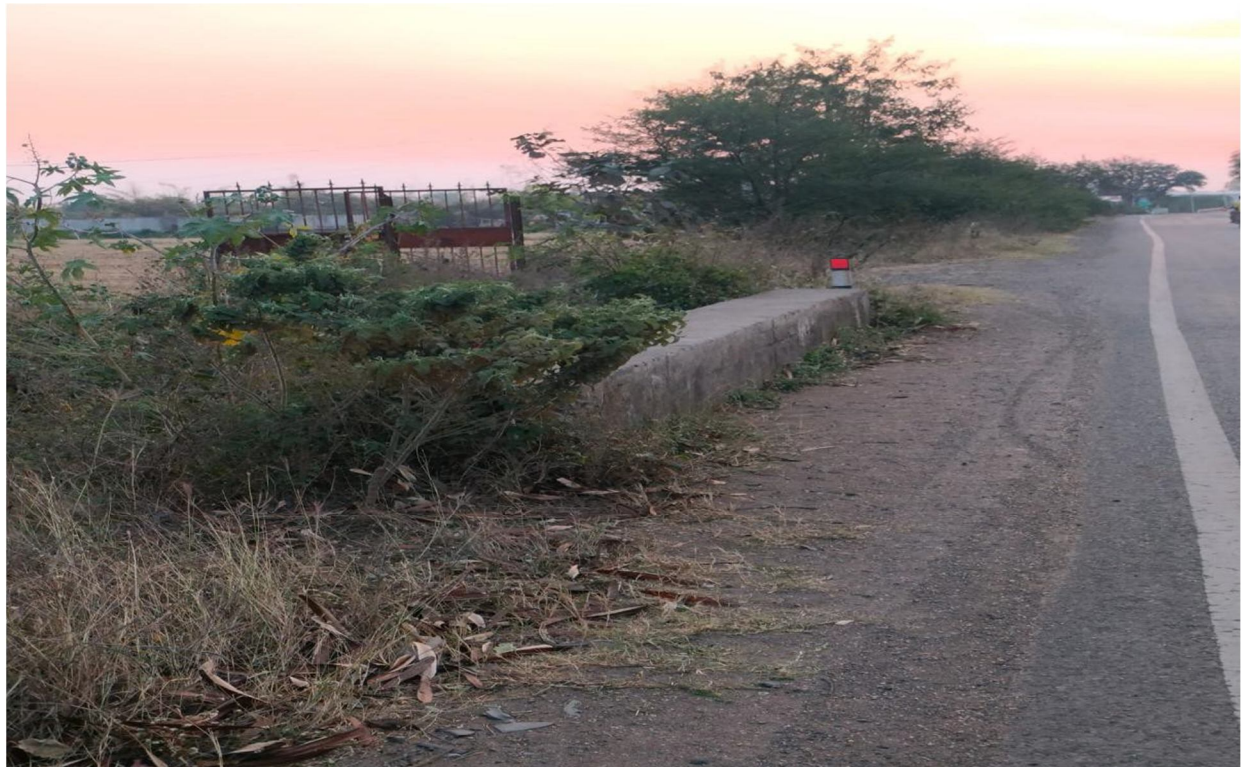
Ch. 17+574 Pipe Culvert Should be painted as per specification
