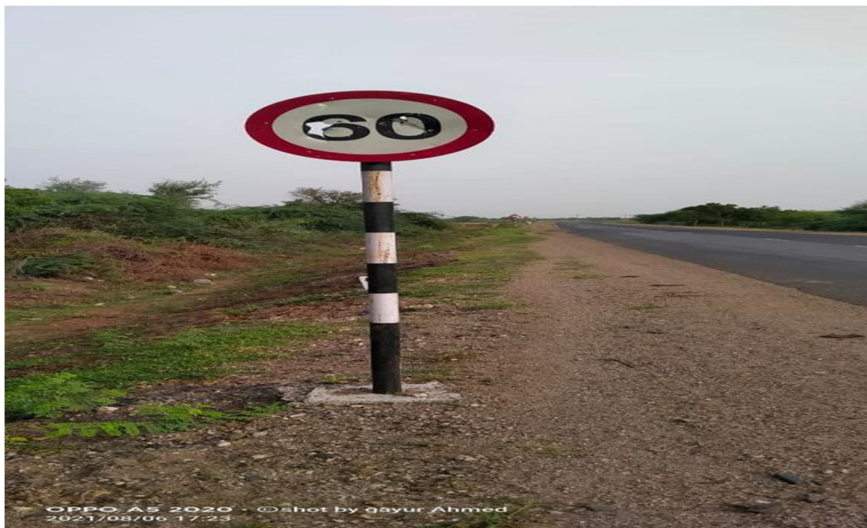
Ch. 26+500 Damaged speed limit sign board
