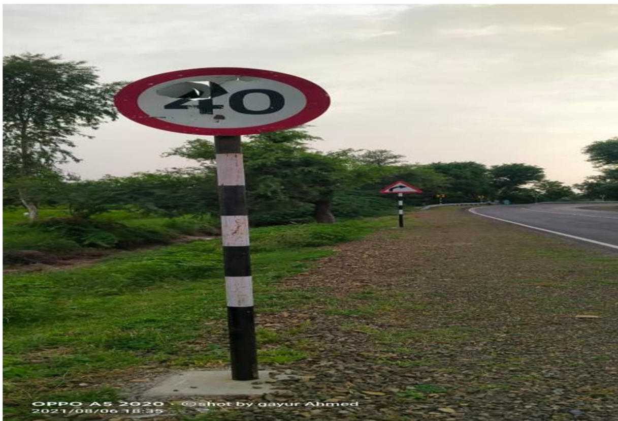
Ch. 16+485 Speed Limit sign board found in damaged condition
