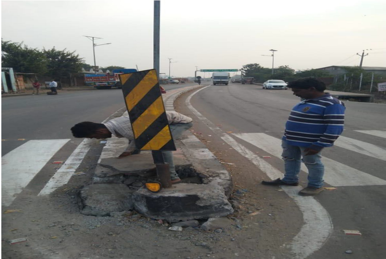
Ch. 0+010 Damaged delineator sign board should be changed & median side kerb should be repaired.
