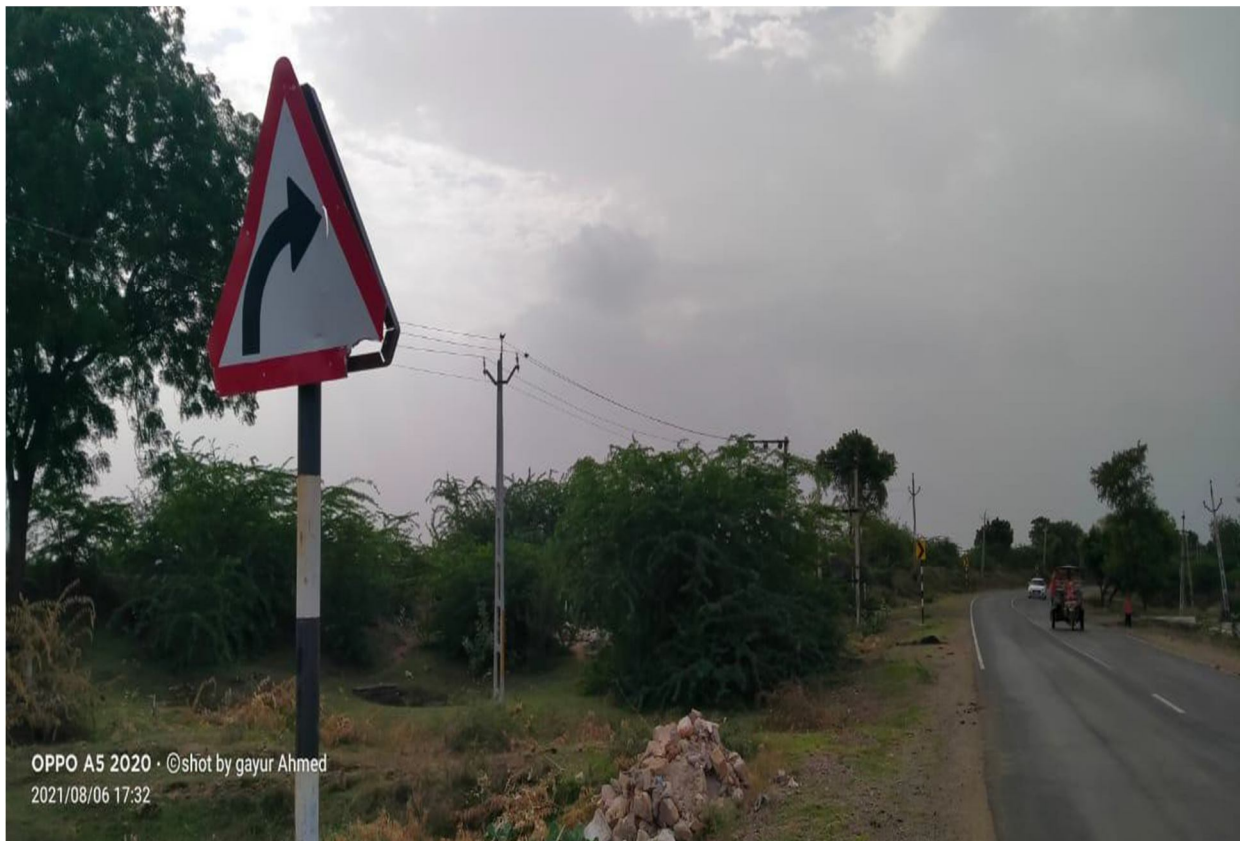
Ch. 3+635 Left turn sign board found in damaged condition & construction material dumped near shoulder
