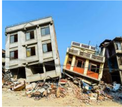
Fig.1 Severe damage on buildings during Bhuj Earthquake (2001)
