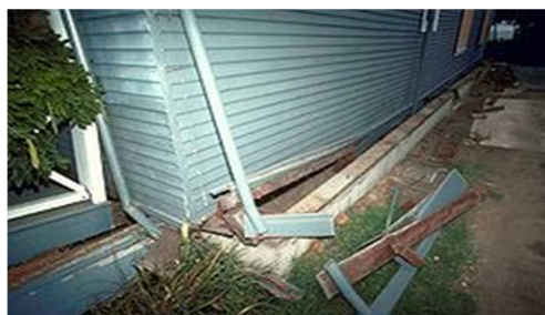
Fig. sliding off failure
