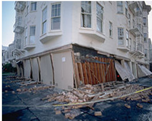
Fig. soft story collapse
