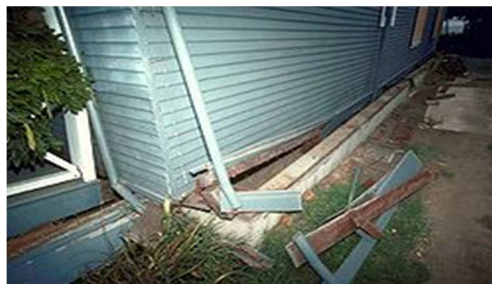
Fig. sliding off failure
