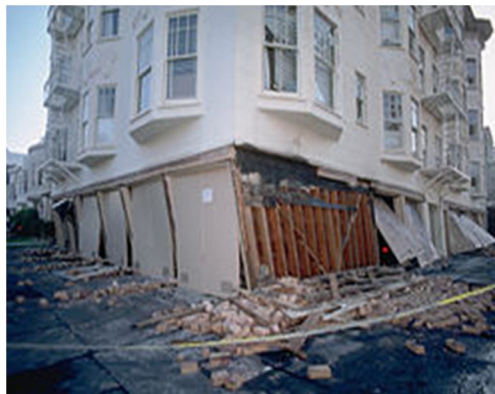
Fig. soft story collapse
