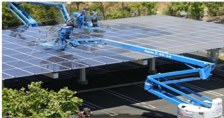
Figure 3 Solar Panel Cleaning Robot
