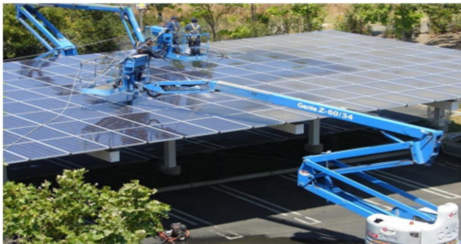
Figure 3 Solar Panel Cleaning Robot
