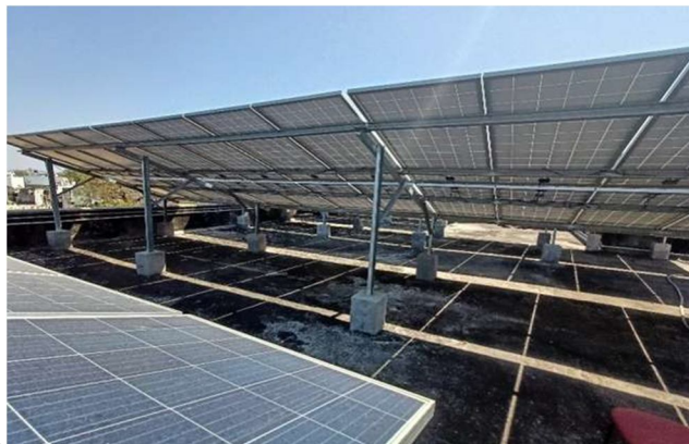
Fig. 1: Solar mounting structure.
