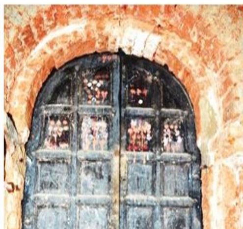
Fig. 2b Details Of Brick Arches Acting As A Lintel For Bearing The Load
