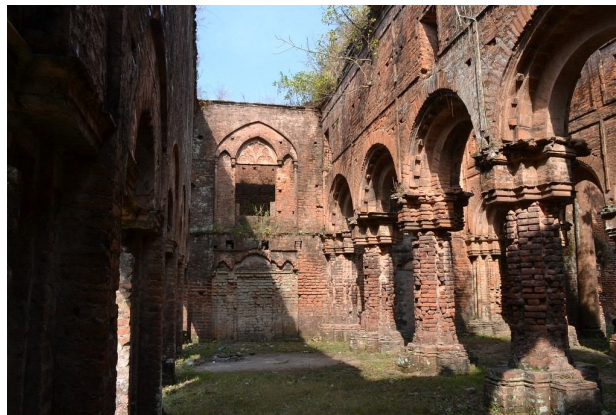
Fig 2a. The Series Of Arches And The Courtyard Inside Tamluk Palace, West Bengal
