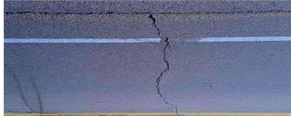
Fig:- Reflection Cracking
