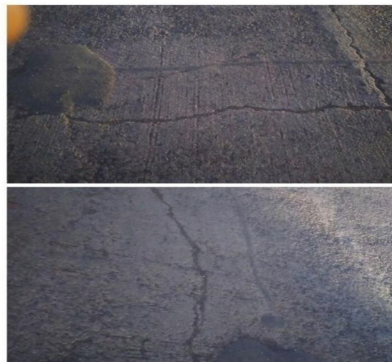
Fig:- Transverse Cracking
