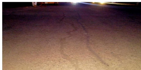
Fig:- Block cracking
