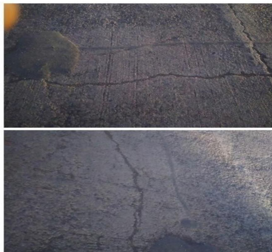
Fig:- Transverse Cracking
