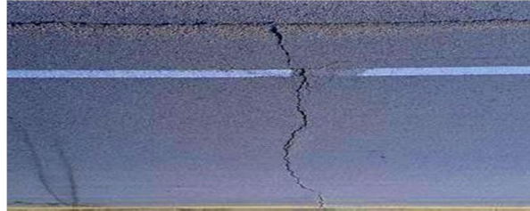
Fig:- Reflection Cracking
