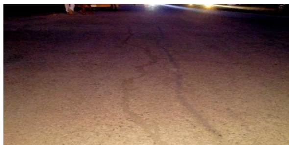
Fig:- Block cracking
