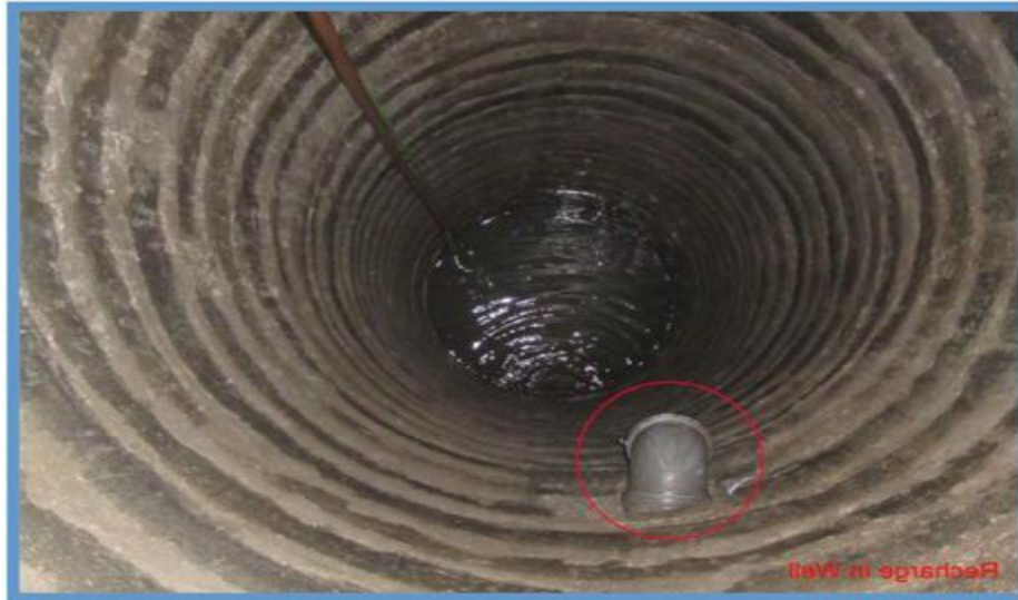
Figure 5 Dug well recharge
