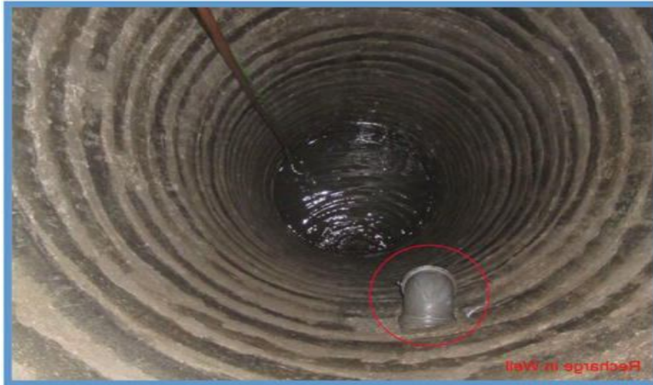
Figure 5 Dug well recharge
