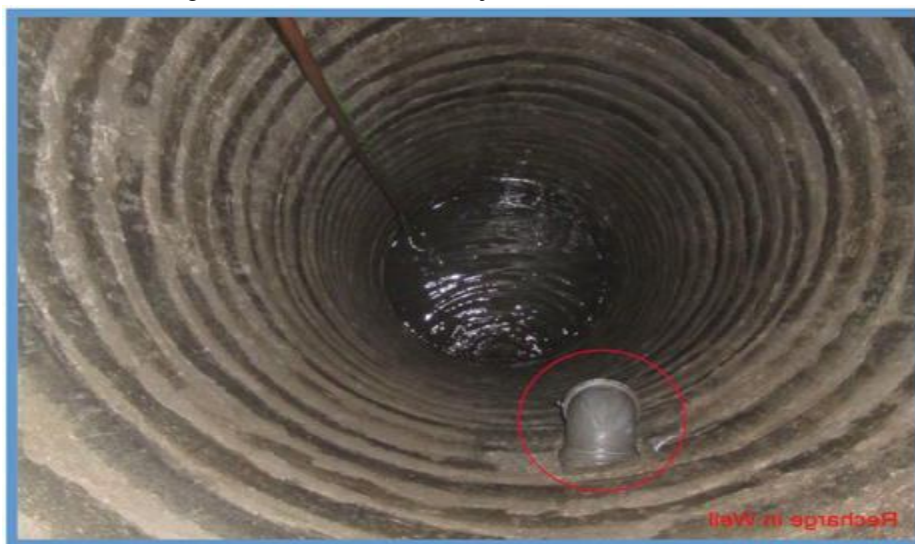
Figure 5 Dug well recharge
