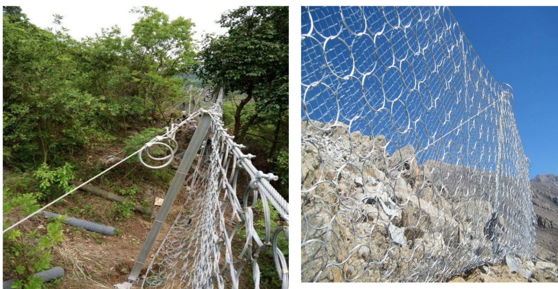
Fig.6:Flexible barrier at the toe of a natural hillside.
