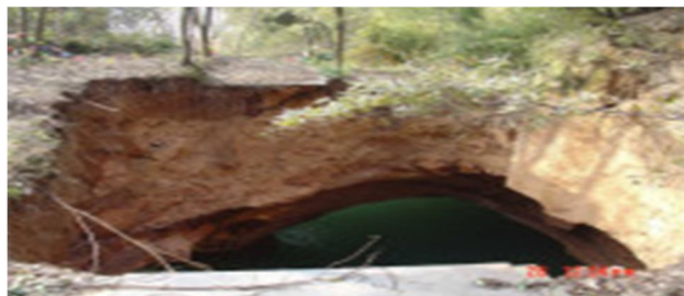
Fig.1. New roof rock collapse with a plane area of 75 m 2 of the originally partially failed
