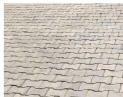
Interlocking paver blocks, allows rain water infiltrate into the ground
