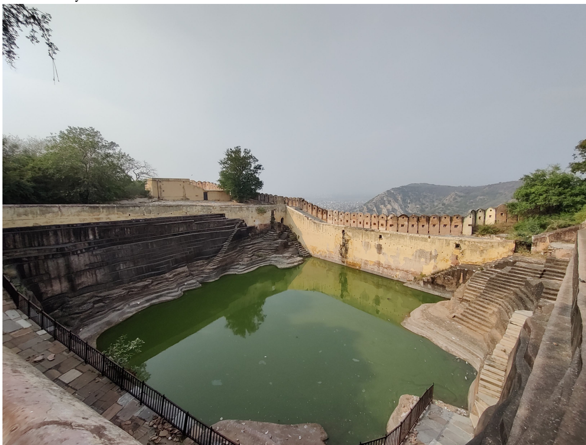
Figure 7: Rain water collecting tanks on fort complex
