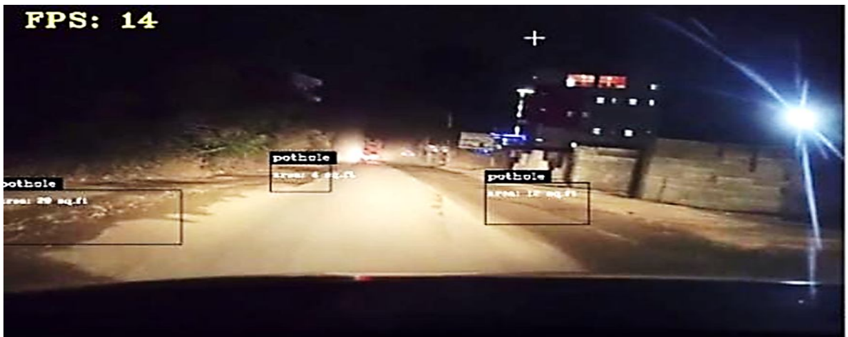
Figure 5: Detection of pothole during night
