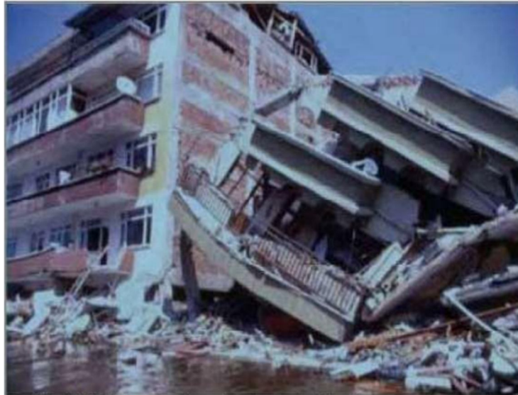
Fig. 1. Multiple-story collapse in a six-story building due to strong beam-weak column design in the 1999 Turkey earthquake.
