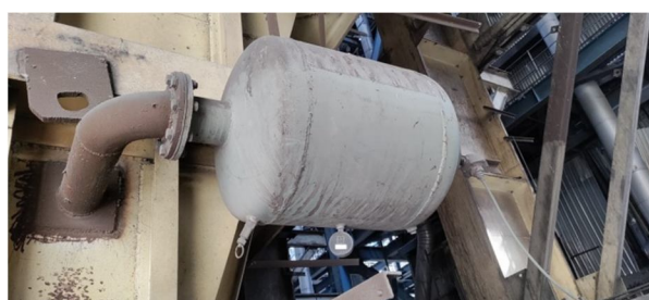
Fig. 3. Air storage Vessel
