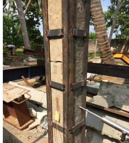
Fig 2: Crack Pattern Showing Buckling
