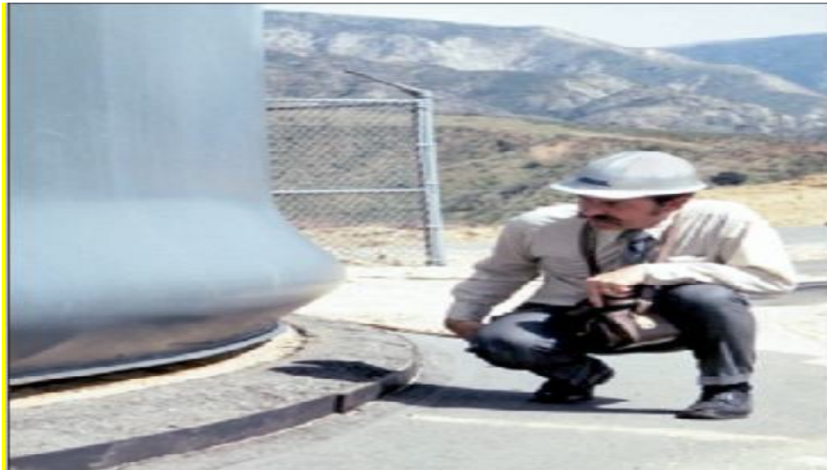
Figure 4: Buckling elephant foot type of tank wall.
