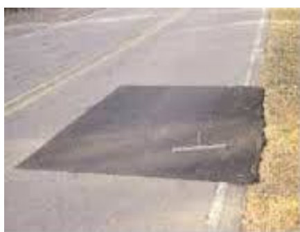
Figure 2 Typical Patched Surface
