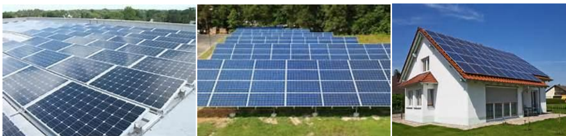
Fig. 9 A photovoltaic system
