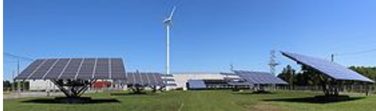
Figure1. Experimental setup – Location of the solar PV panels
