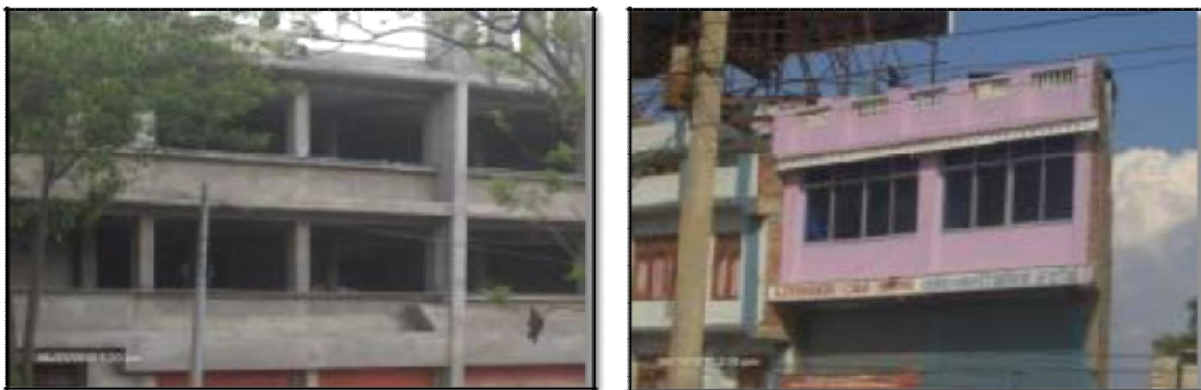
Fig. 1 Partially infilled frames
