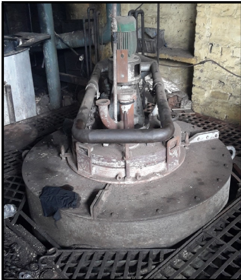
Figure 3. Annealing (gas) furnace
