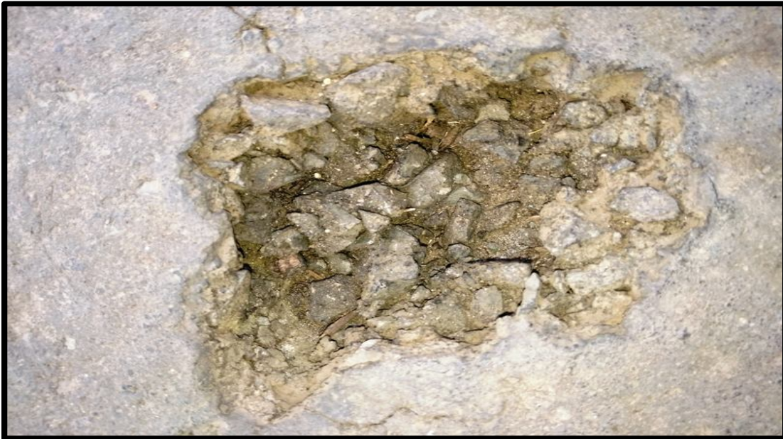
Fig.2 Typical Pot Hole in Pavement before Repairing.
