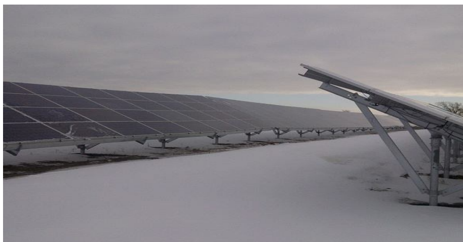
Figure 7. Typical row of solar panels in winter showing very little to no snow accumulation around foundation piles.
