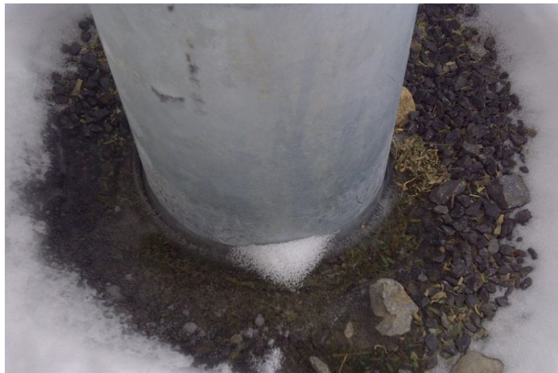
Figure 2. A pile moving out due to frost. The movement can be observed at the base of the pile.
