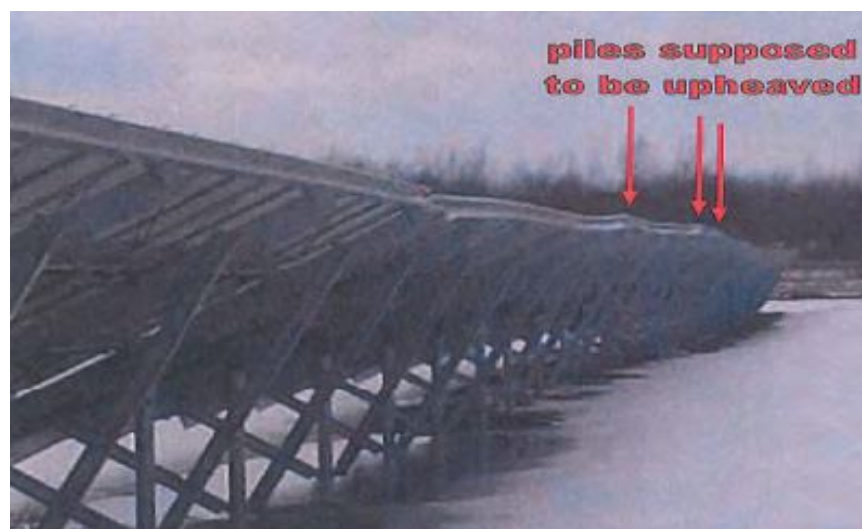
Figure 3. Piles affected by frost showing deformation of the racking.
