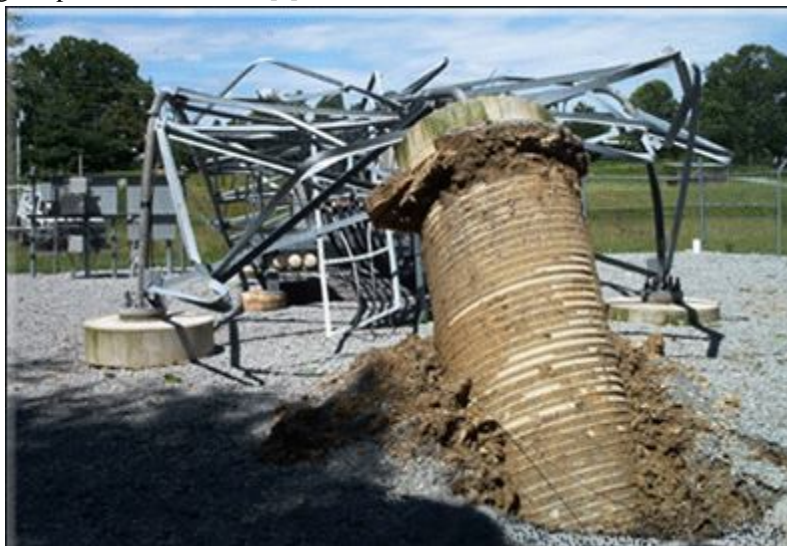
Fig 1:- Tower foundation failing under effects of uplift and frost.
