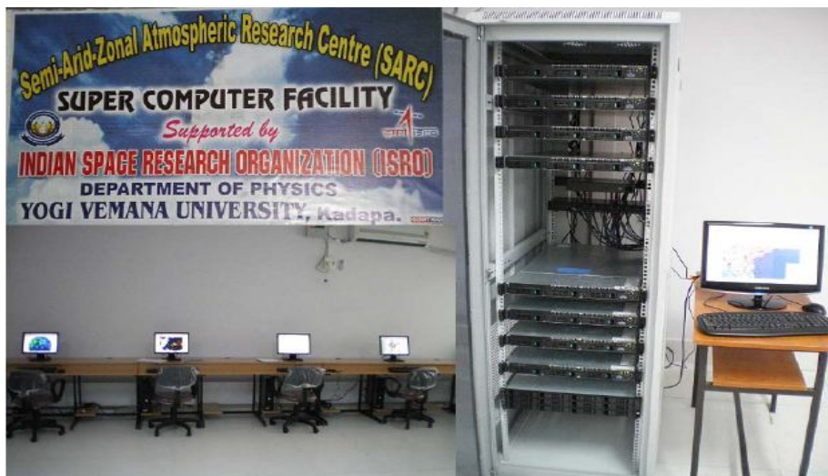
Fig. 3: High Performance Computational (HPC) facility at SARC – Computer (Terminal) room and HPC installed on a rock in a A/C insulated room.
