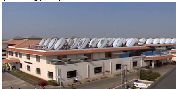
Fig.4.2 solar cooking system
