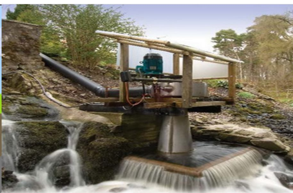
[Fig 12: Power production through SHP Plant]
