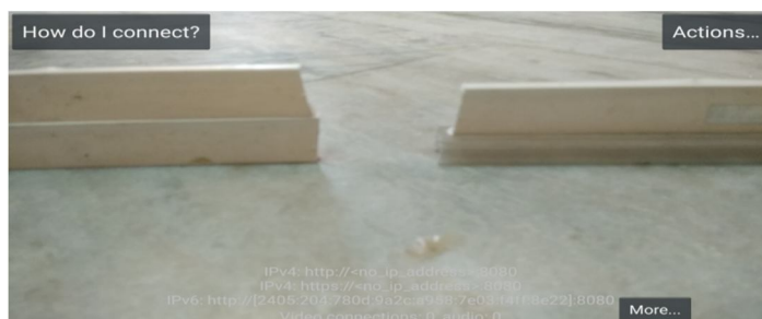
Fig.7 Screenshot of live-video streaming of the crack
