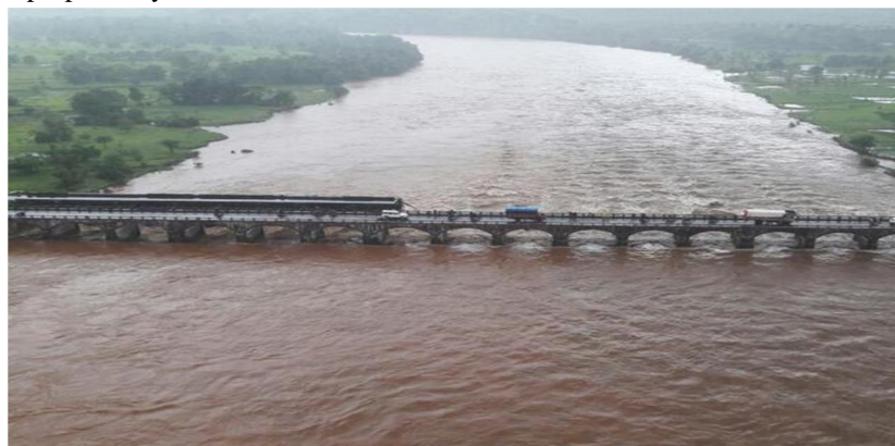
Fig 6. Bridge Collapsed due to heavy rain.
