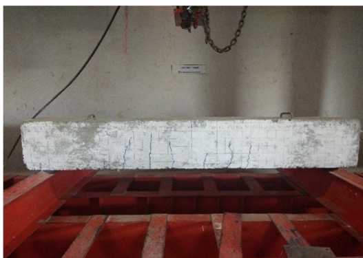
Figure 7 Crack Pattern after loading
