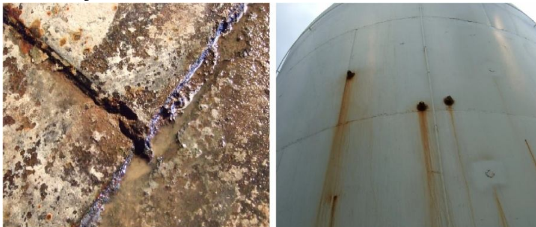
Fig. 1 Evidence of Shell Corrosion [13]
