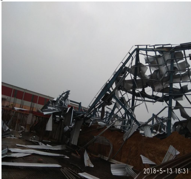
Fig. 3 Structure failure due to storm in Delhi [Image courtesy to client]
